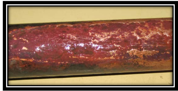
Fig.2. Pitting corrosion of tube wall,
